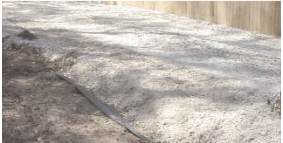
The Mirafi® HP370 permanently stabilized easement supports the heavy water trucks and operational equipment.
