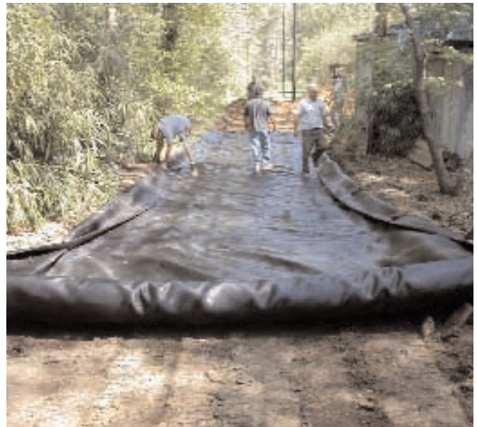
This project required a high strength geotextile due to the weak soils and perched water table.
