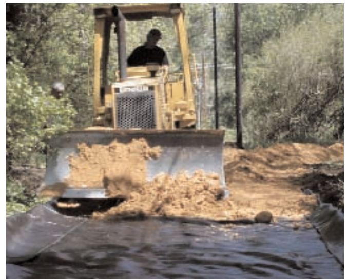
By using a geotextile, costs were minimized by using the existing ground fill.
