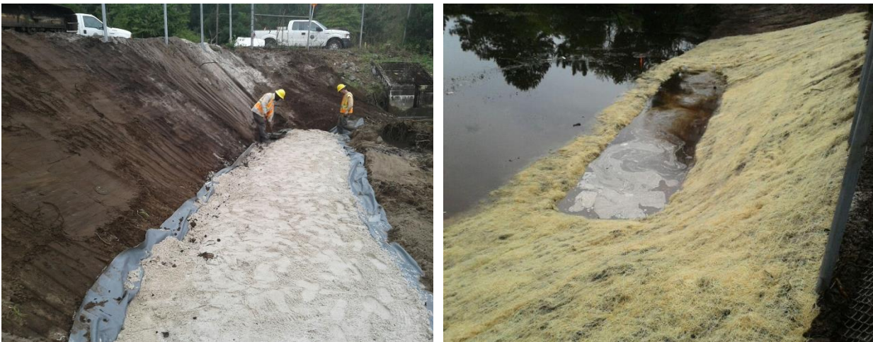
Figure 6. Littoral shelf filter during construction (left) and following a rain event (right).
