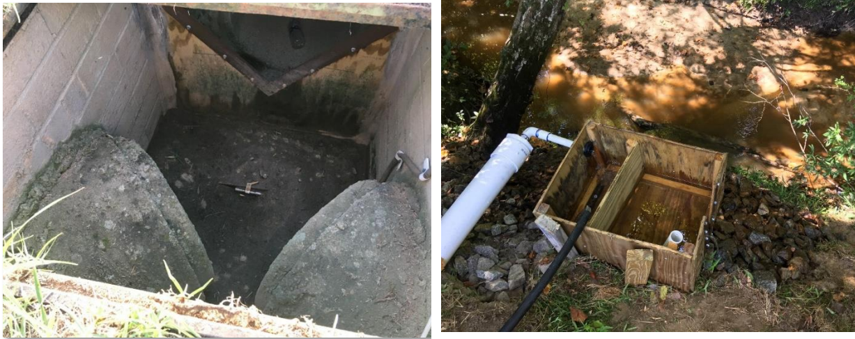
Figure 7. Monitoring equipment installed at the inlet of Sapphire pond (left) and filter underdrain at Bridgewood (right).
