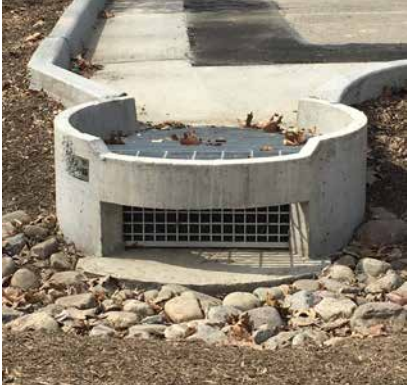
Concrete chamber for residential & urban sites
